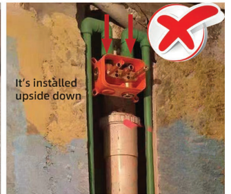
It's installed upside down The installation of concealed plastic box in wrong way
